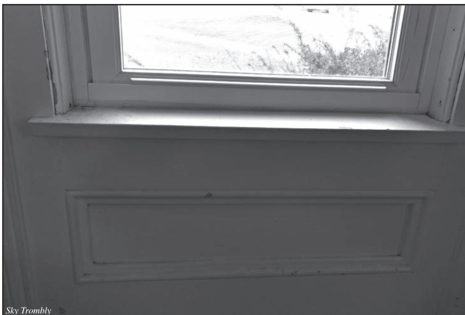
The use of lead based paints in houses in the U.S. was banned in 1978. Many older houses still contain these paints and this is a common source of lead poisoning in children. Photo Sky Trombly
