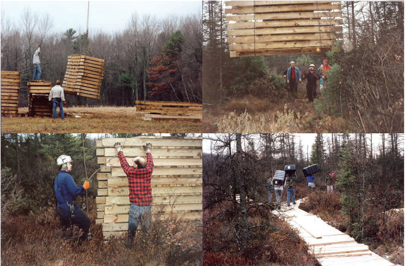
Stacks of boardwalk sections were attached by cable to the helicopter. They were flown to the bog and detached while the helicopter hovered overhead. The sections were then joined together on a system of floating drums. Images courtesy of David Buck
